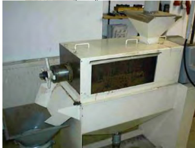
expeller presses (leakages / lub)
