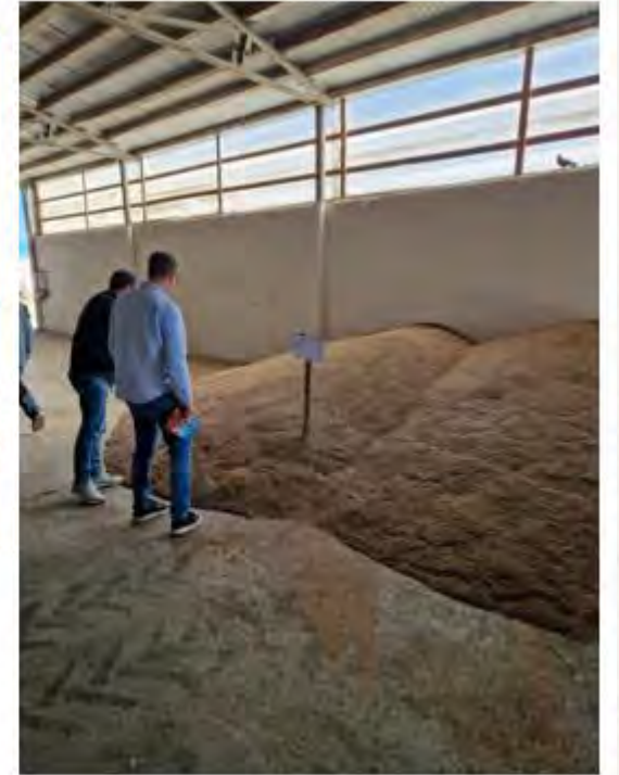
leakages on the concrete-floor contact with asphalt-floor?
