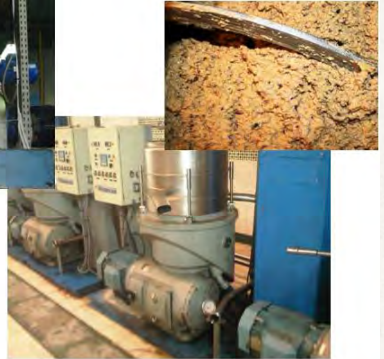
lubrification of malaxeurs /presses (leakages)
